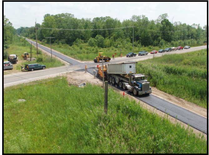
Construction crews build a new stretch of the Wadhams to Avoca Trail.
