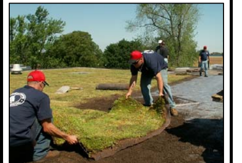
Workers install vegetated mats of sedum on the Fine Arts Building roof of SC4.
